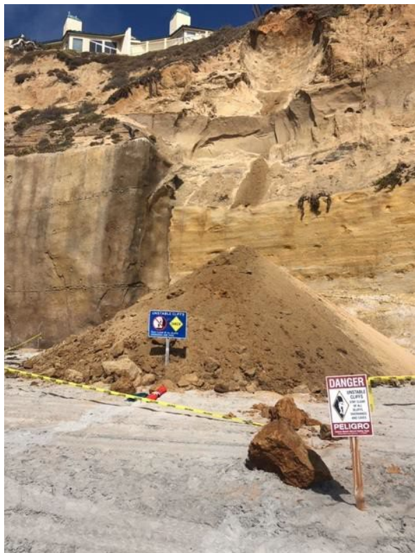
Figure 4-2: Bluff Collapse in Solana Beach September 13, 2019
