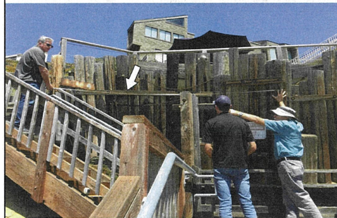
PHOTO 2: NORTHERLY C-CHANNEL WITH TIEBACKS TO BE LOCATED BELOW EXISTING WOOD WALER (ARROW).
