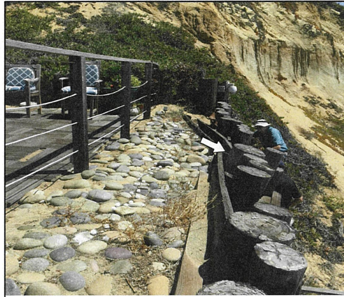
PHOTO 1: NOTE POLE WALL LEANING SEAWARD.
