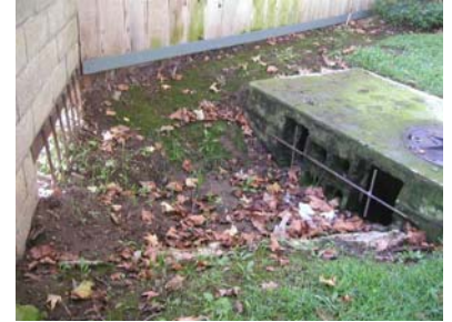
Earthen swale with inlet
