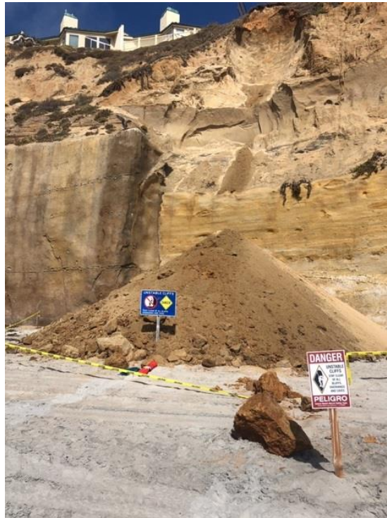
Fig. 2 Bluff Collapse in Solana Beach September 13, 2019
